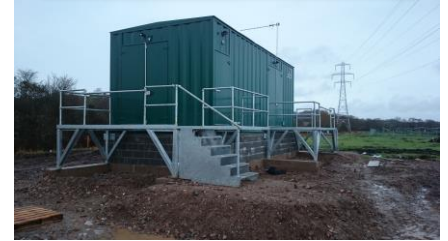
WPD/JUWI Combined Substation
