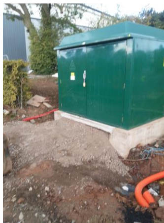
WPD / SSE Substation
