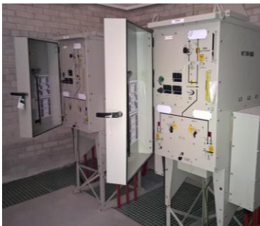
SP 1000kVa Package Substation
