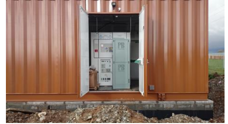
WPD/JUWI Combined Substation
