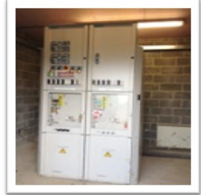
33kV Siemens Switchgear with the overcurrent protection and surge arresters
